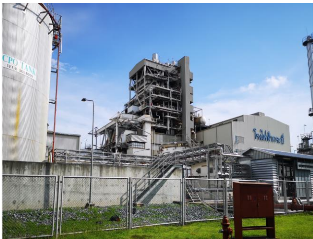
Fig. 4. Krabi power plant.
